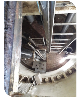
After: Shaft entrance Long-range lighting
