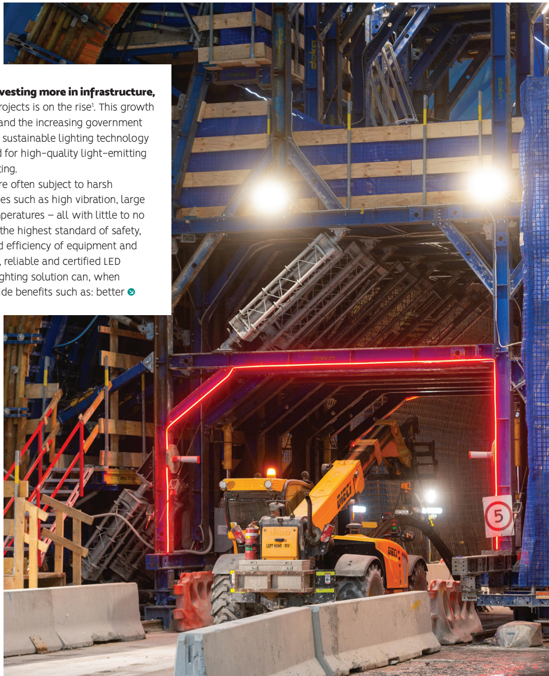
Above: Cross River Rail using red LED Strip lighting ALL IMAGES COURTESY: MINEGLOW
